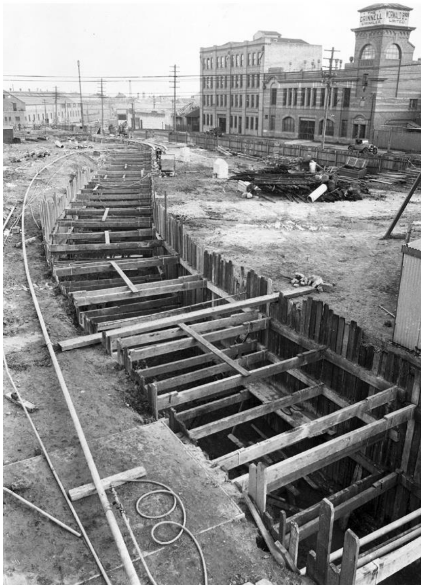
Figure 29. Formwork for construction of underground stormwater channel feeding into the Alexandra Canal, Waterloo 3 August 1928 (Contributed By City of Sydney Archives [67311] (Sydney Water 'A' Series Photographs A546)
