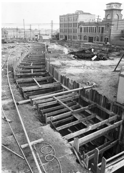
Figure 26. Formwork for construction of stormwater channel underground in Waterloo 3 August 1928 (Contributed By City of Sydney Archives [67311] (Sydney Water 'A' Series Photographs A546)
