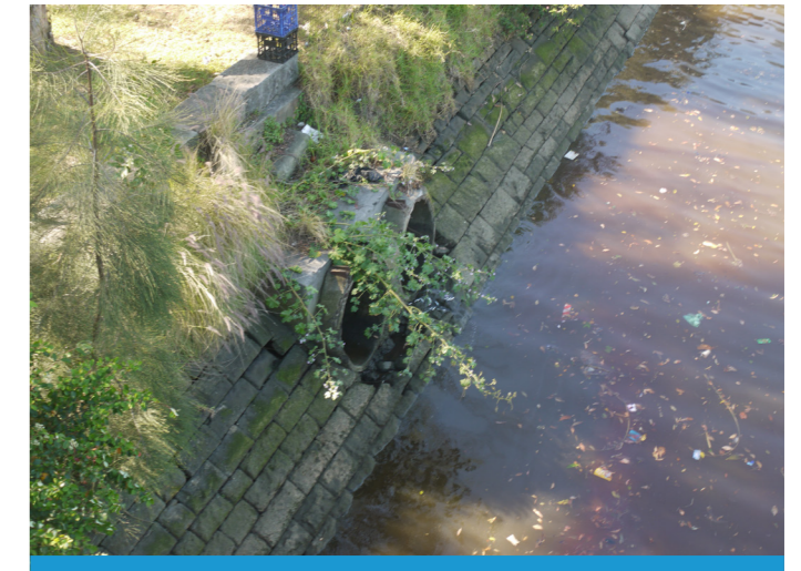
Figure E-9 - There are a few existing stormwater outlets into the canal within this section. This have been co-located at various points along the river, such as the location shown in this image.
