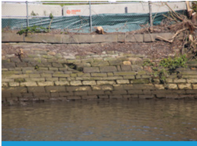
Figure E-18 - Section of eastern wall in the vicinity of the proposed Bridge 10.
