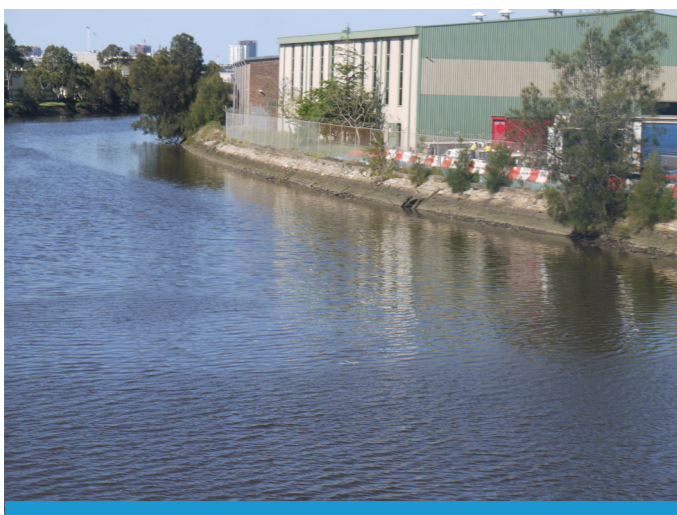
Figure E-6 - Alexandra Canal is a large open span of water with earthen banks lined by primarily sandstone blocks. The wall has been modified at various sections with different materials, however the Archives reach remains primarily intact.
