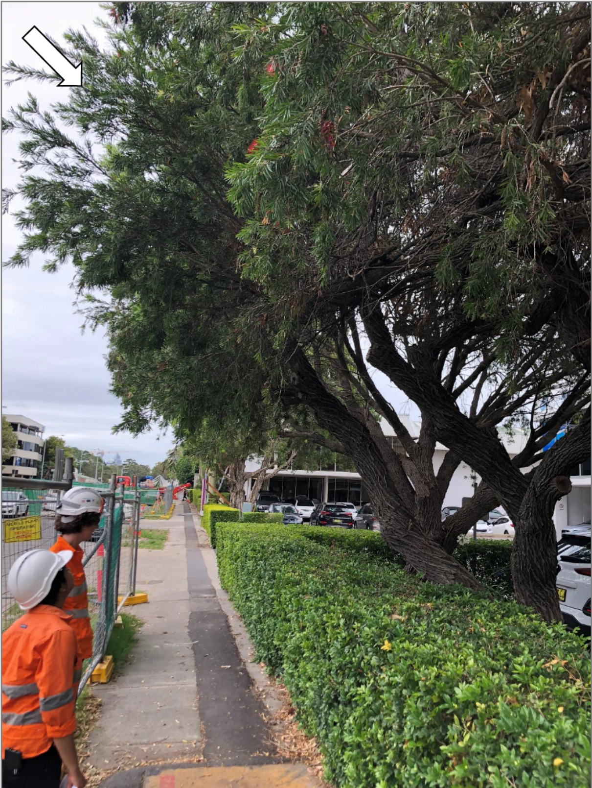
Plate 5 – A2 147 & A2 151s – Weeping Bottlebrush – Arrow note limbs requiring removal to accommodate light pole installation/positioning.
