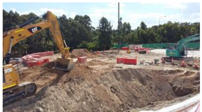
Earthworks to prepare the area for the tunnel shaft at the Bexley Road south construction site, January 2017
