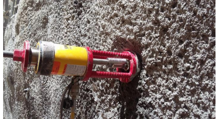
Installation of rock bolt in the shaft to support the tunnel structure at the Bexley Road north site, January 2017
