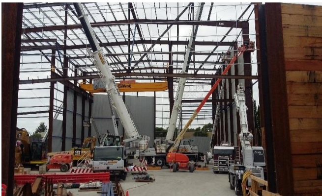
Construction of the acoustic and spoil shed at the Bexley Road north site, January 2017
